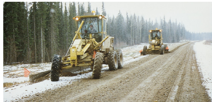
Slow, controlled grader operation is key to reducing culvert inlet and outlet damage. Reduce damage by keeping graders on the road running surface. Never side-cast gravel toward culvert inlets or outlets.
