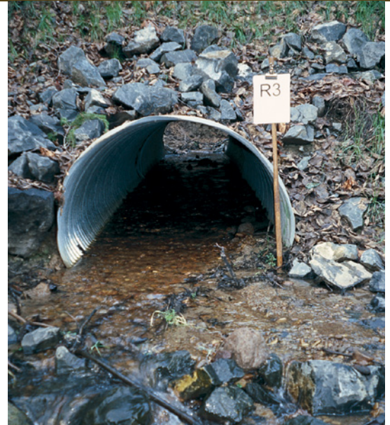
A round galvanized corrugated metal pipe sunk into the streambed to allow for fish passage.
