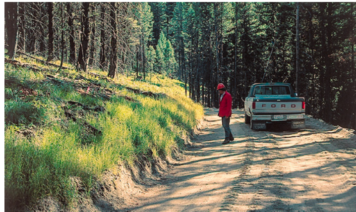
Grader damage to inside ditch toe slopes exposes an easily erodible surface and is a source of sediment.
