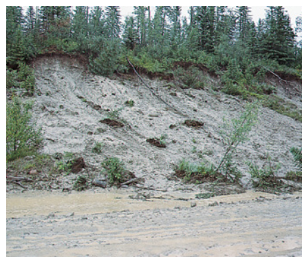
Poor road surface drainage caused this fill-slope erosion.
