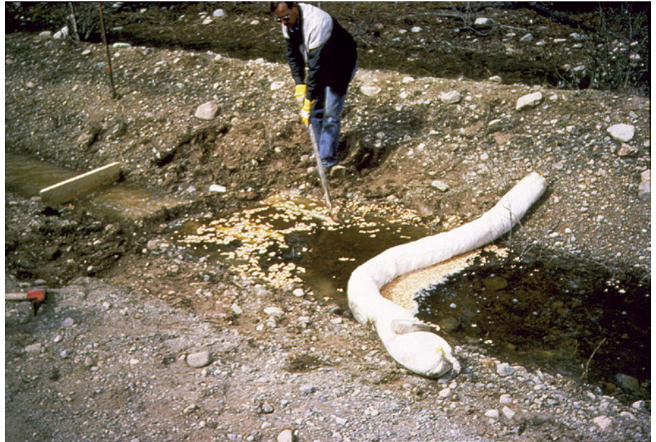
Spill kits are used to contain hazardous materials.
