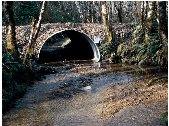
Arch culvert on a low-clearance road, sunk into the streambed to allow for fish passage.
