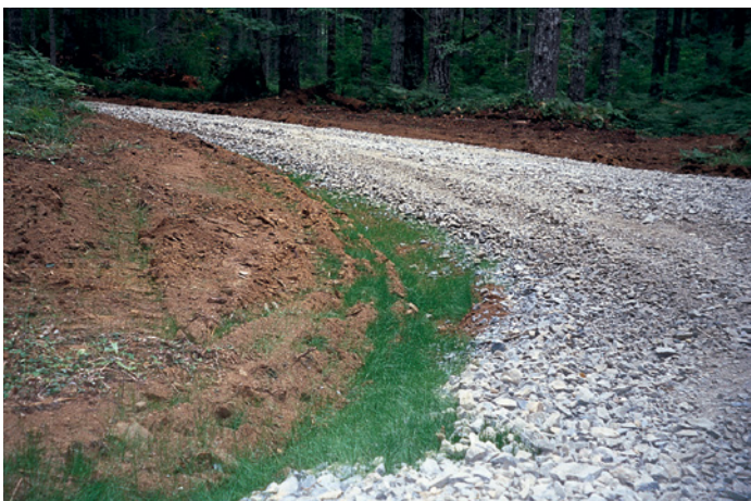
Road surfacing can double the cost of a road. However, gravel roads can provide all-weather access, reduce road maintenance costs and protect water quality by covering the soil with a weather-resistant surface.
