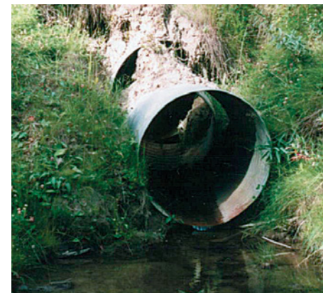
Watch for damaged culverts that need replacement. Repair work should be completed during dry weather.
