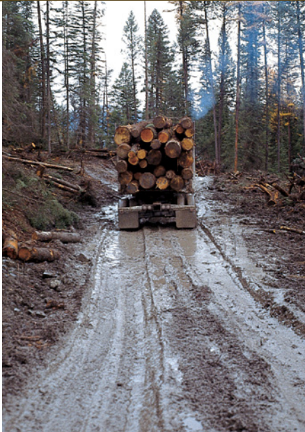
Roads receive heavy use during logging. Be aware of early signs of damage. Serious damage to road surfaces starts with excess water. Standing water is a sure sign of road-drainage problems. Ruts indicate that road strength is deteriorating.
